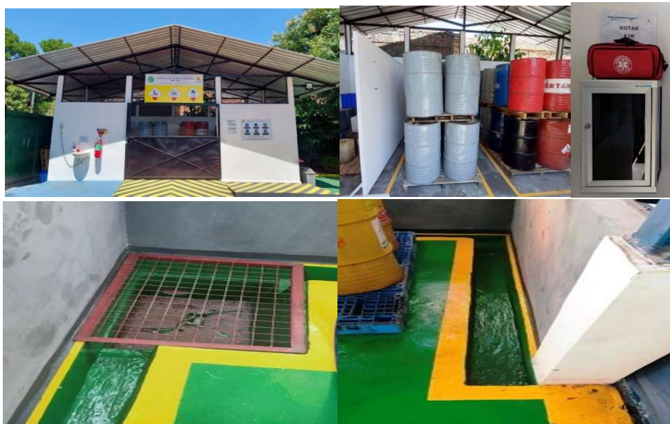
Figure 10. Hazardous Waste Storage
