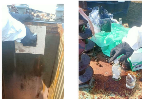
Figure 9. Transformer Offline Oil Sampling for PCBs Test
