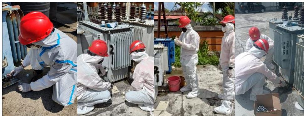
Figure 7. Transformer Offline Oil Sampling for PCBs Test
