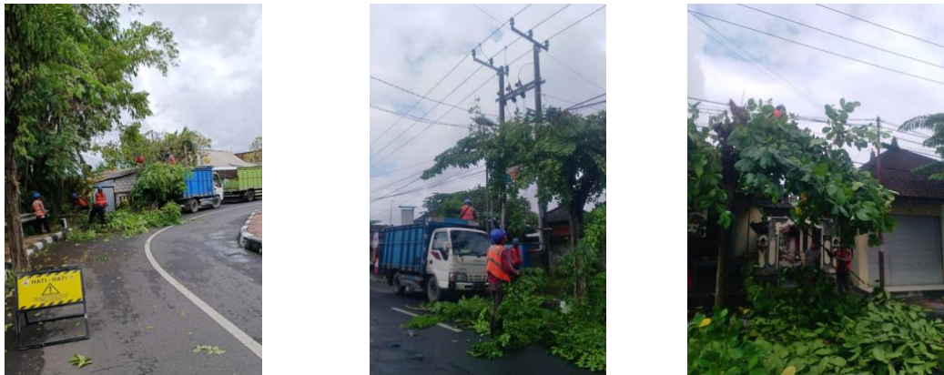
Figure 3. Tree Trimming Around Power Lines
