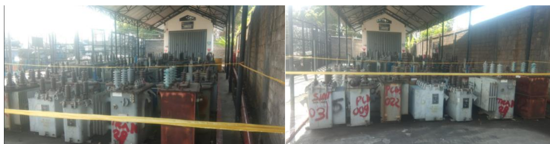
Figure 8. Transformer Containing PCBs Storage Area
