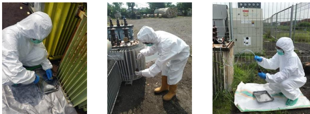
Figure 6. Transformer Offline Oil Sampling for PCBs Test
