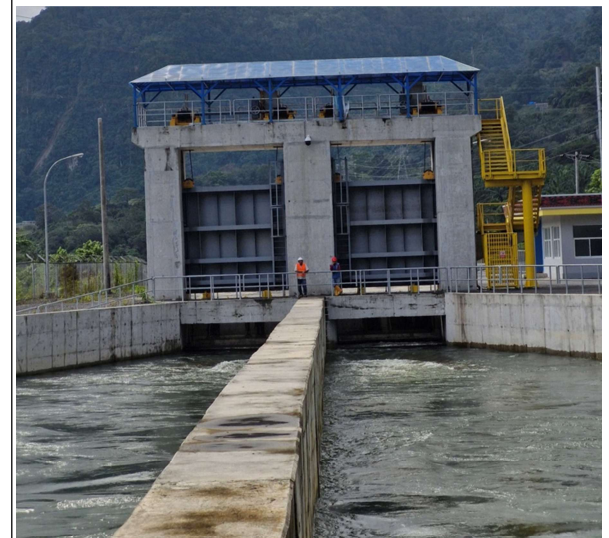
Photo 66: Headpond sand flushing gates
