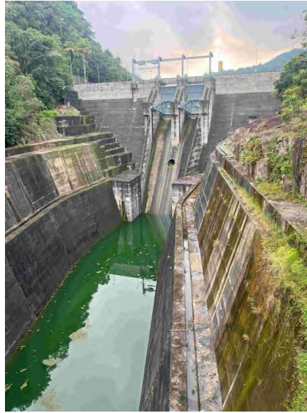
Photo 8: Siguragura dam, part of Asahan-2 project, with no release of maintenance flow
