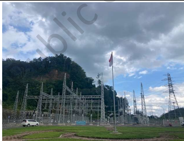
Photo 35: Switchyard next to control building
