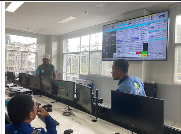
Photo 36: Control room displays
