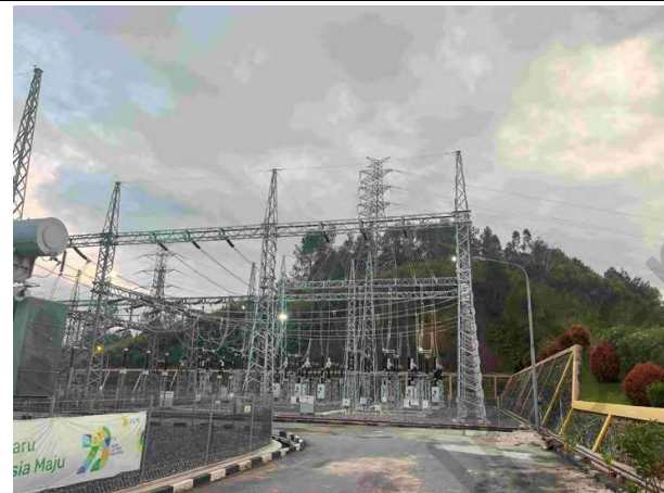
Photo 4: Simangkuk substation, end of transmission line from Asahan-3 HPP
