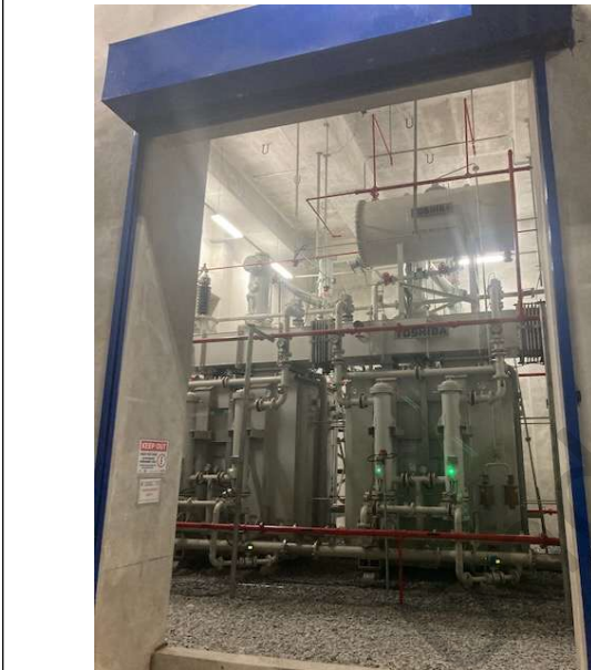
Photo 40: Transformer bay in powerhouse
