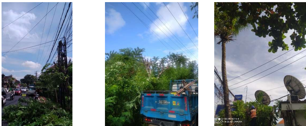
Figure 3. Tree Trimming Around Power Lines
