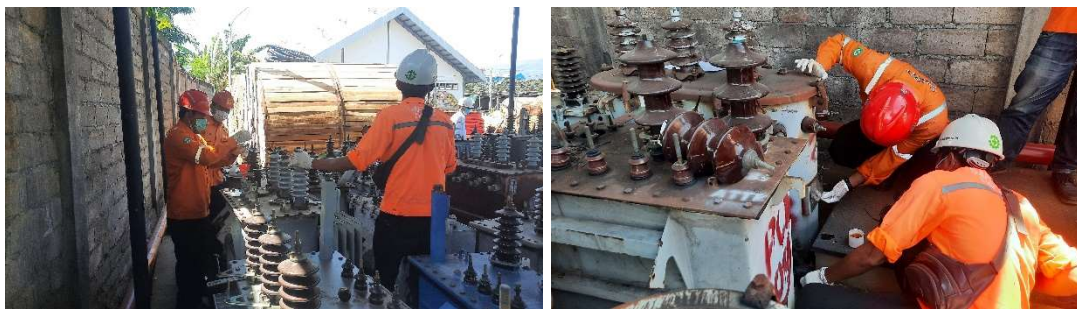
Figure 7. Transformer Offline Oil Sampling for PCBs Test
